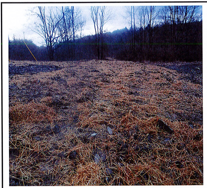
Straw mulch does not meet stabilization standards.
