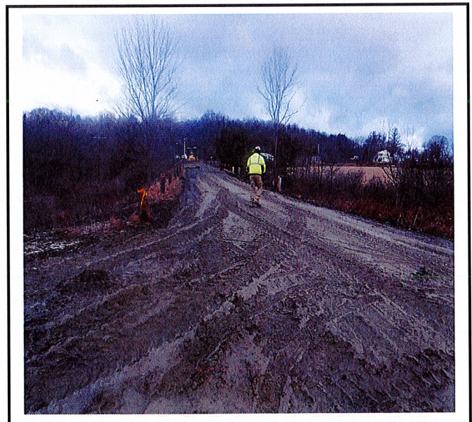
Road into substation many inches thick of mud.
