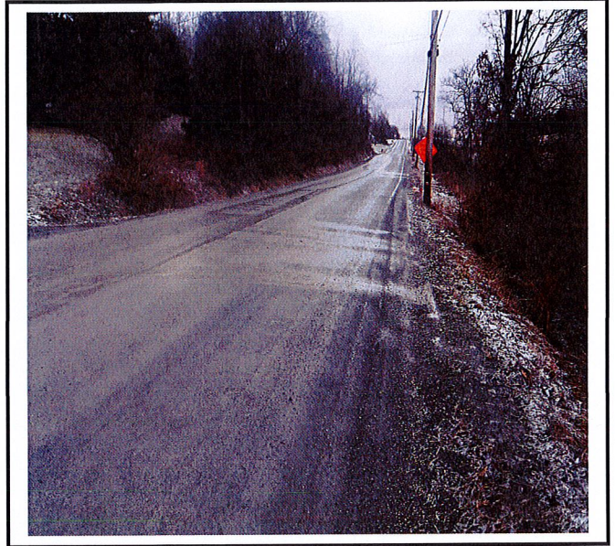
Rain has caused sediment tracked from site to runoff road.
