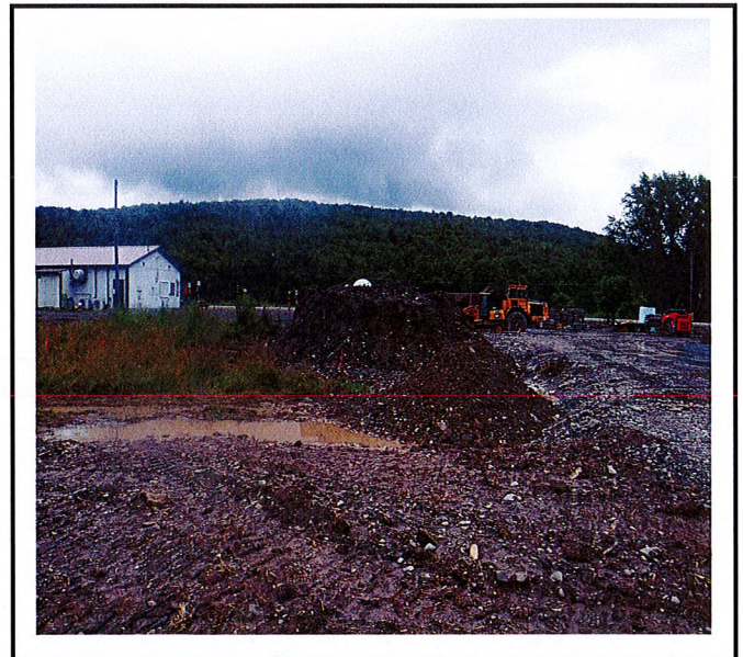
Topsoil stockpile does not have stabilization or straw bales and silt fence surrounding it as approved SWPPP indicated.
