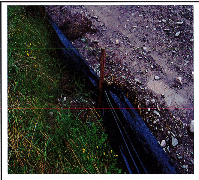
Silt fence requires repairs in many areas. It is ripped off stakes and had holes in it.
