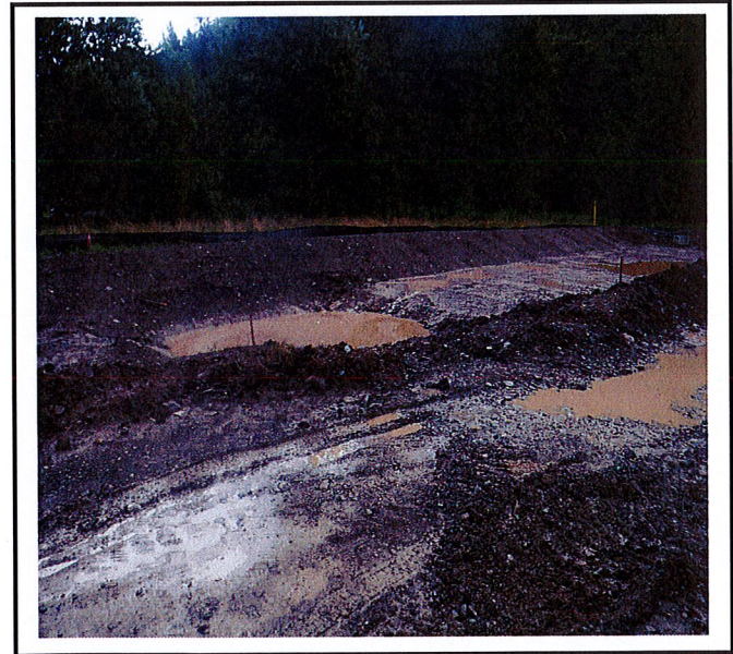
Rock outlet protection hasn't been installed as part of the sediment trap.
