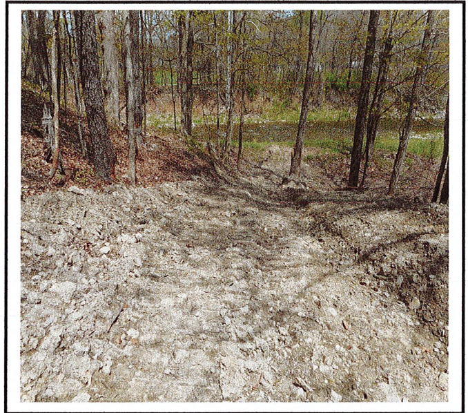
Swale discharges directly to Bentley Creek. Erosion and sediment controls should be installed ASAP.
