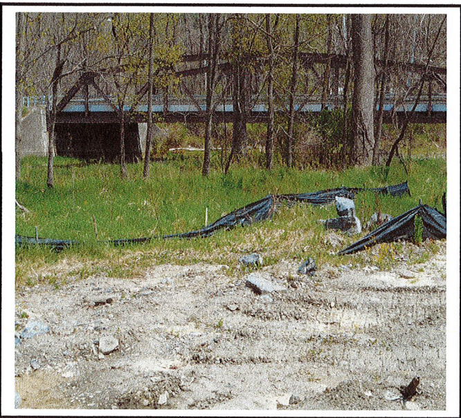
Silt fence will need to be replaced before work begins again.
