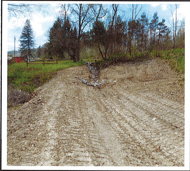
Swale constructed on the west side of the project requires erosion and sediment controls.
