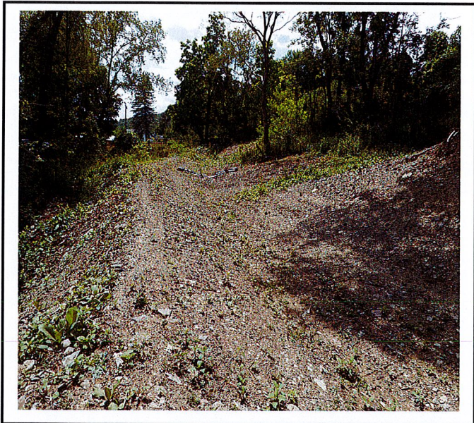
Rock check dams and stabilization not installed in diversion swale.
