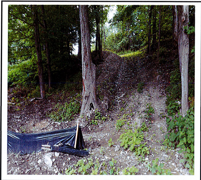
Slope protection matting not installed in diversion swale.
