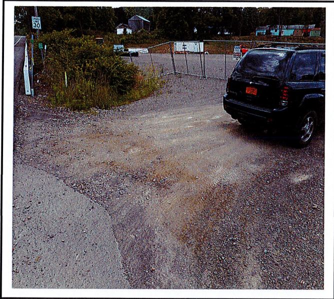
Construction Entrance needs to be installed.
