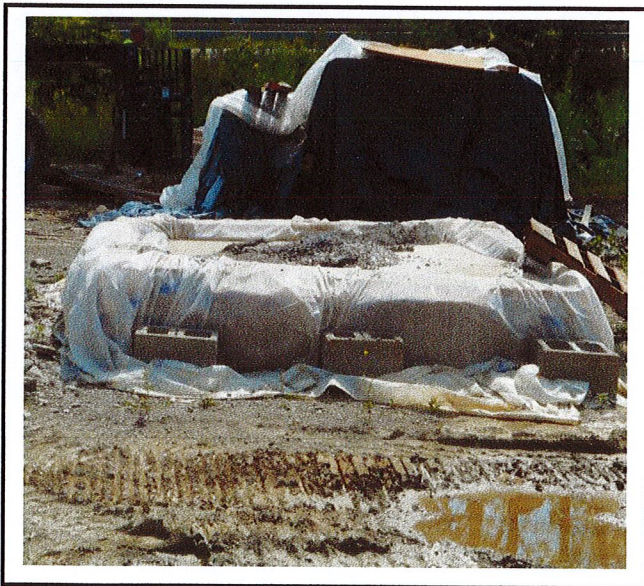
Concrete washout requires replacement.
