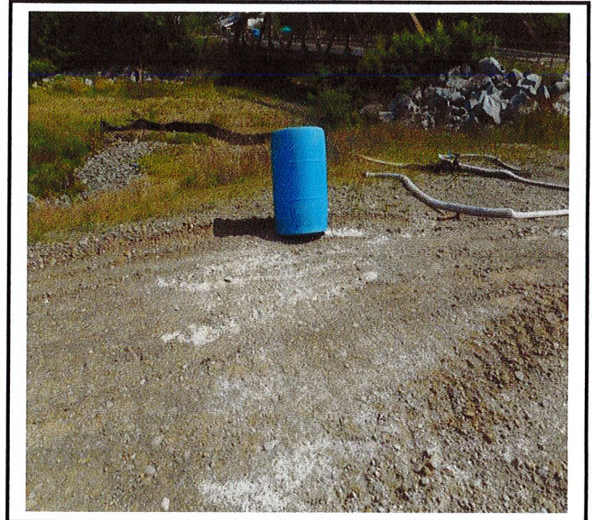
Barrels and mortar mixing should not be washed onto the ground.
