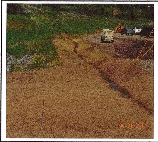
Stormwater channel on the south end of property has been installed and stabilized.
