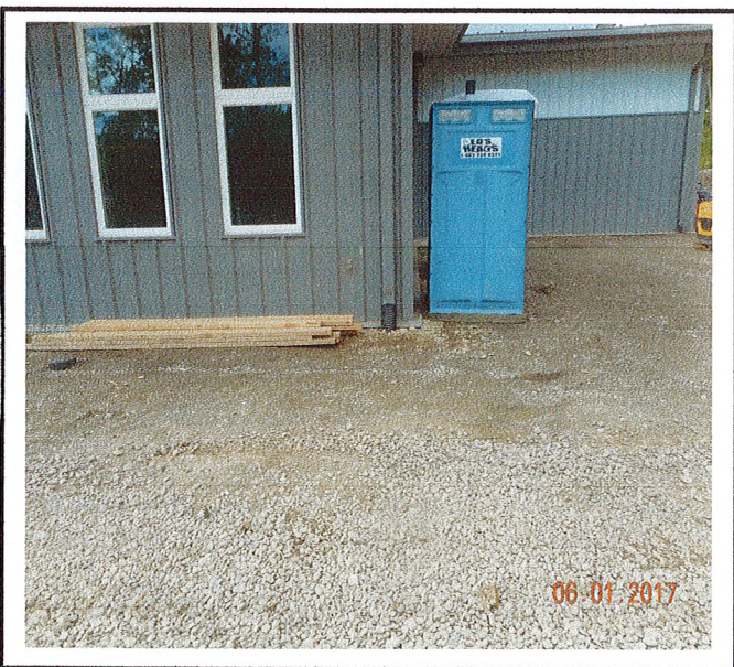
Roof drains have been tied into the stormwater system.
