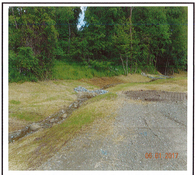
Conveyance ditch has minor erosion.
