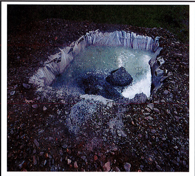
Concrete washout almost at capacity. Plastic is ripping on sides.
