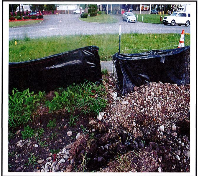
Silt Fence not correctly spliced together.
