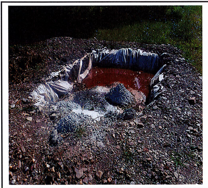
Concrete washout requires replacement. Plastic liner is ripped and soil is exposed.
