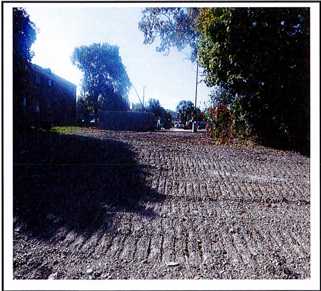
Drainage swale does not look like it has been established to the stormwater pond.
