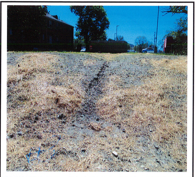
Erosion in the drainage from dumpster pad down to pond needs to be repaired.
