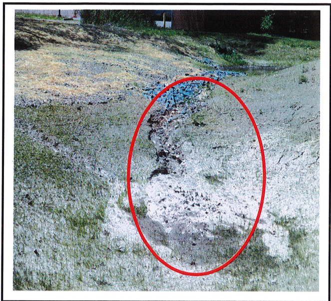
Erosion has occurred in the rock wier overflow. Erosion needs to be repaired and sediment removed.
