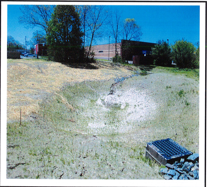
Soil stabilization over the entire pond is needed.
