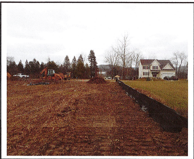
Silt fence has been installed but needs to extend to all areas shown on approved plans.
