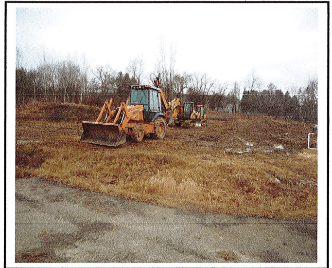
Silt fence has not been installed at this location.
