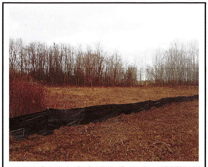
Clearing of trees and brush has occurred in two areas outside of the approved plan. This is not acceptable.
