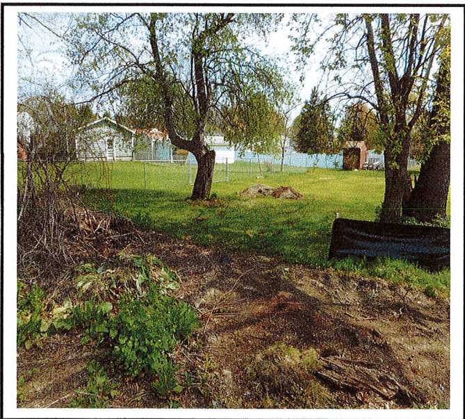
Silt fence does not extend past disturbed area. Neighbor is dumping yard waste at project site.
