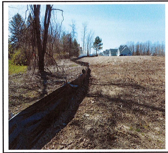
Bare soil areas require stabilization.
