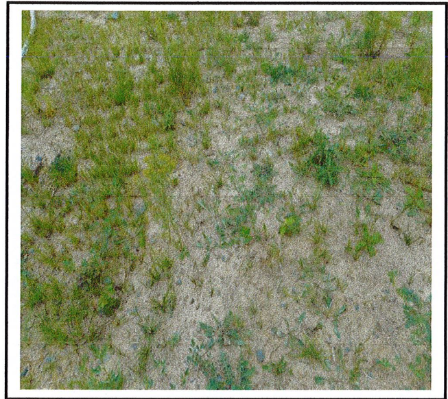
Temporary stabilization is not adequate.
