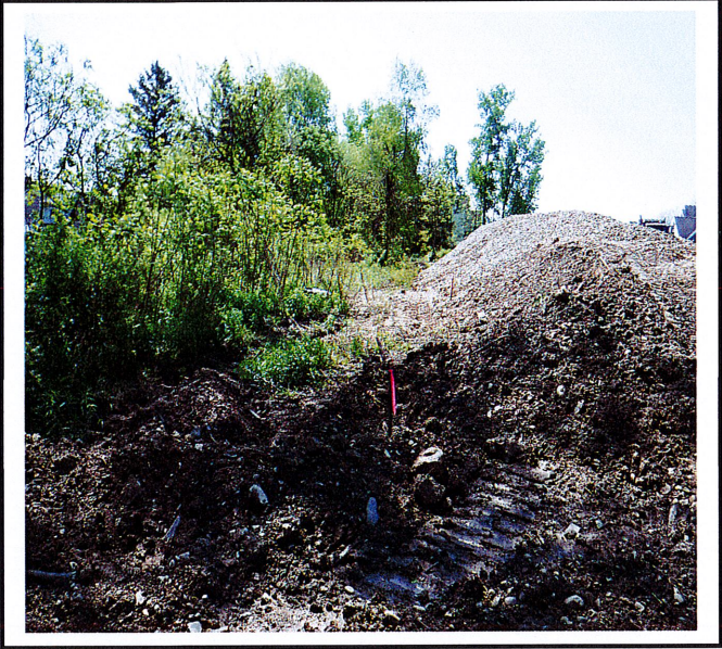
Silt fence is not installed at the toe of the slope between house lots and stormwater basin.
