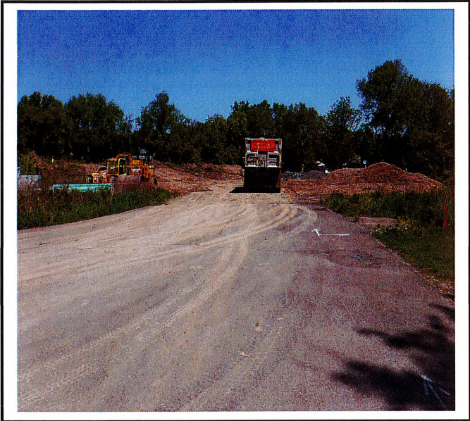
Construction Entrance requires maintenance.
