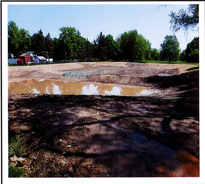
Stormwater Basin has been constructed. Recent rain events have caused erosion on the side slopes of basin. Forebay has taken substantial sediment.
