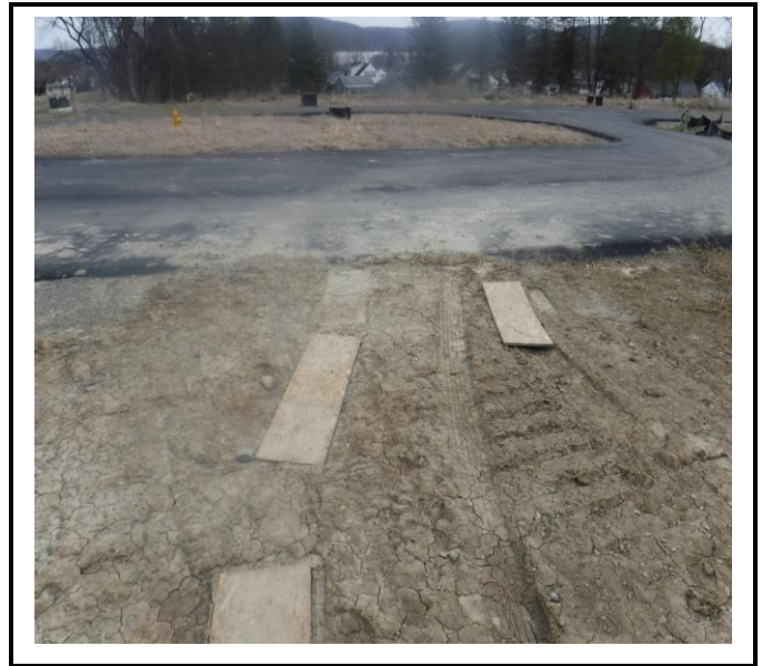
Vehicles accessing property outside of the limits of disturbance AND no construction entrance. You can see evidence of mud tracking onto the road.
