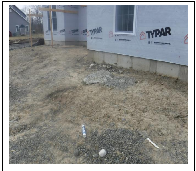
Concrete washout is all over the open lots. There is not one concrete washout on the open lots or any other.
