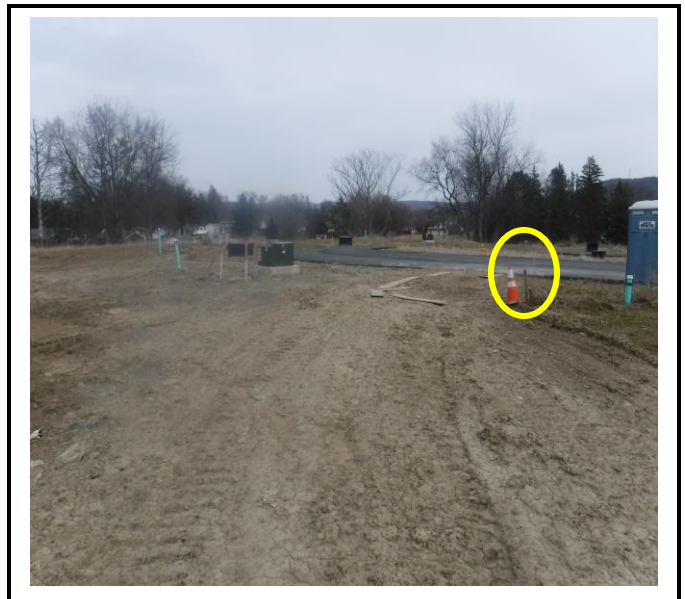
Work continues outside the limits of disturbance. These other lots are not approved for any disturbance at this time. See lot stake marker.
