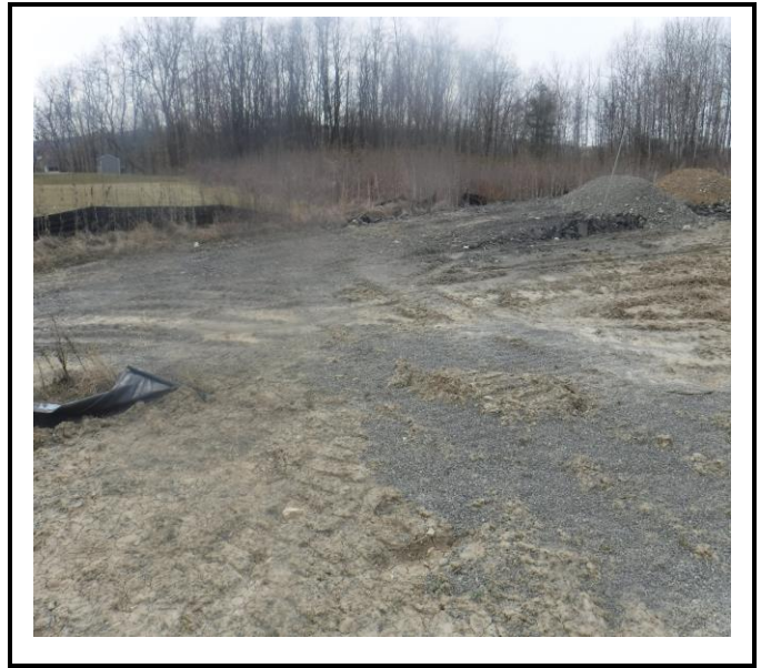
Construction Entrance- traffic is only supposed to enter and exit through stabilized construction entrances. Traffic is still bypassing these areas and tracking.
