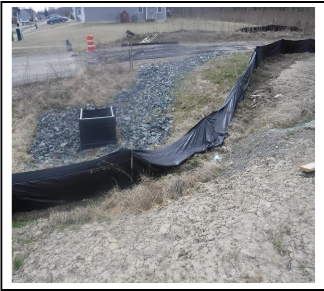
Silt fence- many areas of silt fence need replacement or maintenance.
