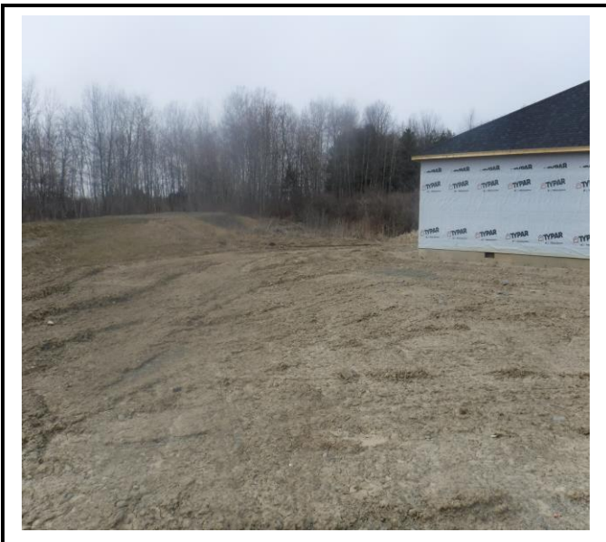
Soil stabilization- Any area that has bare soil not being worked for longer than 14 days requires stabilization. This soil has been exposed for months.
