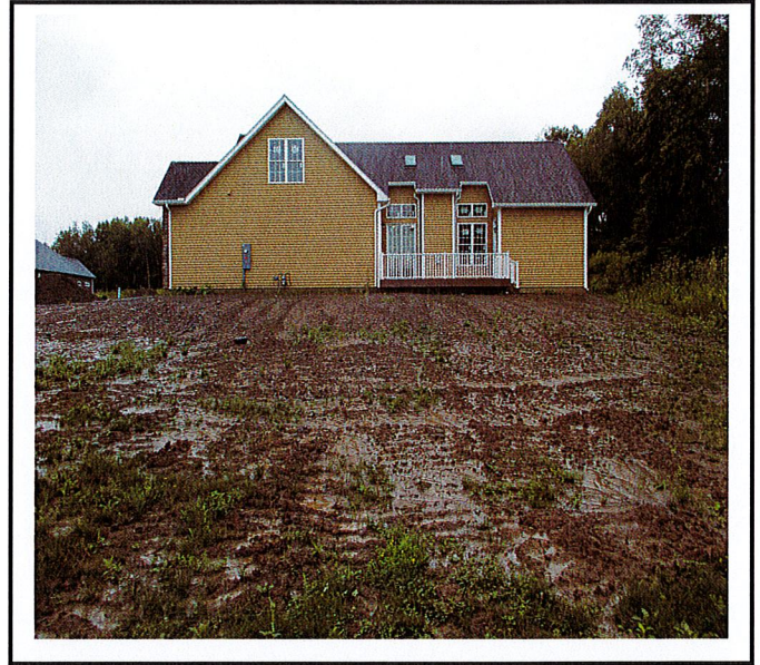
Lot #6 is the only lot under construction. The E&S plan is not being followed and all of this exposed soil is getting mixed with stormwater and going to basin.
