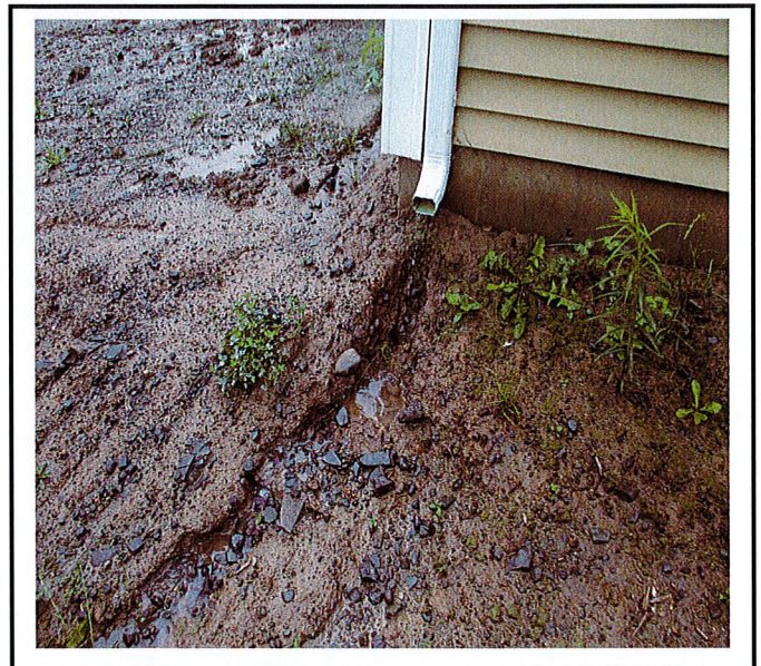
Downspouts directed onto bare soil are causing erosion around the entire property.
