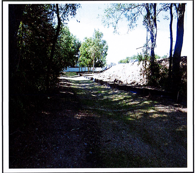
Swale along south end of Phase 1 is growing grass and been stabilized.
