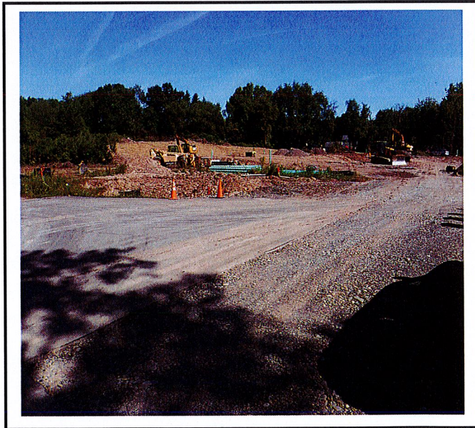
Construction entrance may need maintenance soon.
