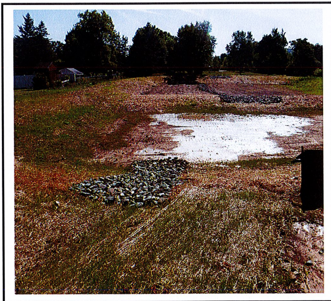
Stormwater forebay and retention basin.
