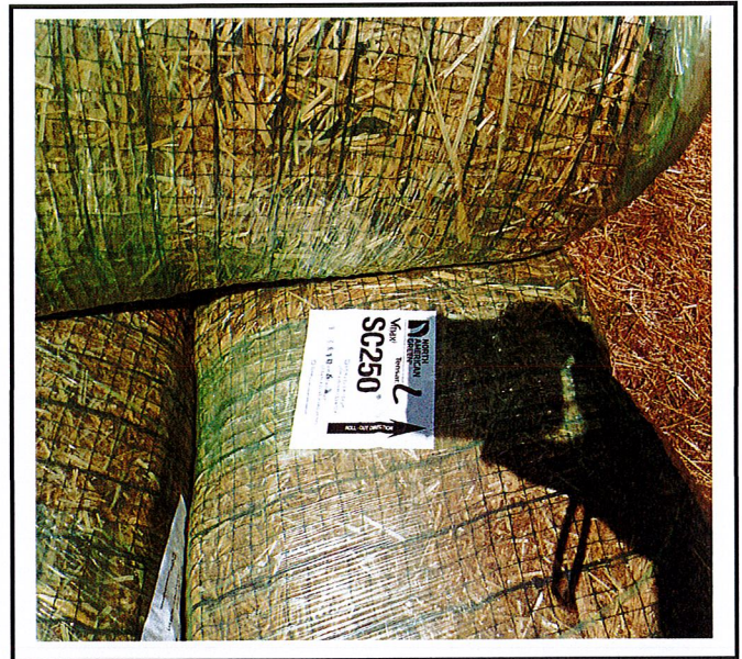
Turf Reinforcement Mat (TRM) on site for swale on north end of property.
