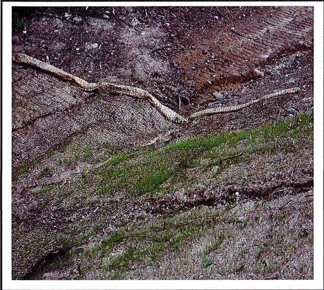
Erosion has occurred on the side slopes of the north drainage swale.
