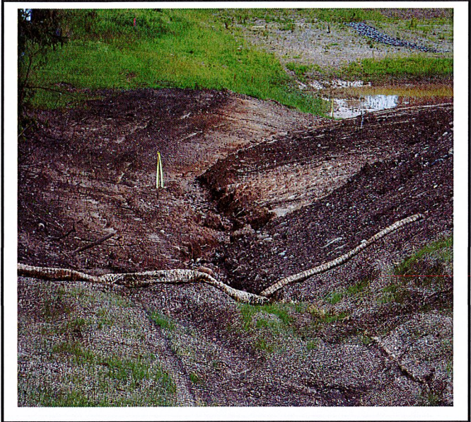
Erosion has occurred in the center of the swale where the erosion control blanket ends. The erosion has headcut under the blanket as well.
