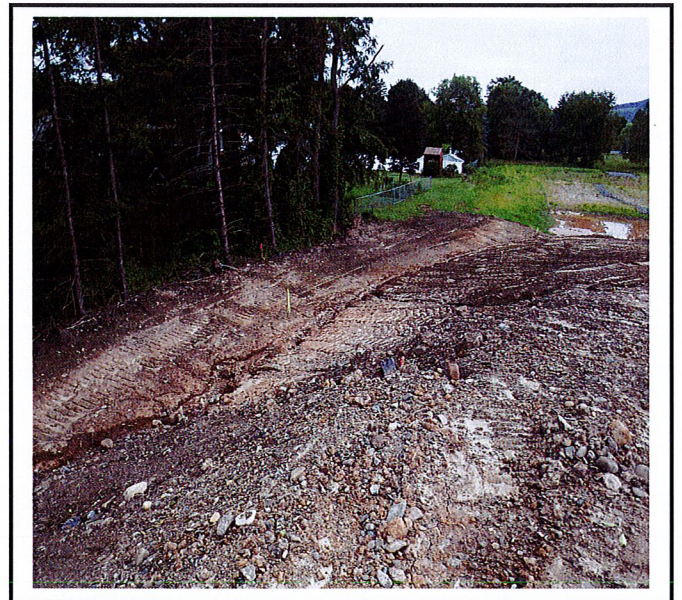
Erosion of the drainage swale along the North end of the property occurred where erosion control blanket was not installed.
