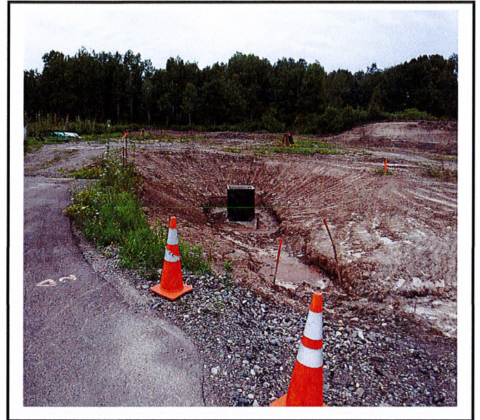
Erosion has occurred around the catch basin closest to Lynhurst Ave.
