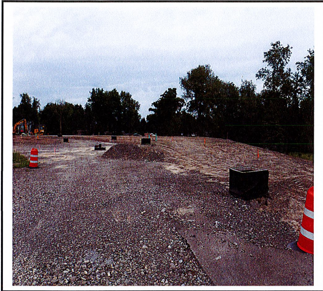
Site is being graded and storm sewer has been installed. All catch basins have protection.
