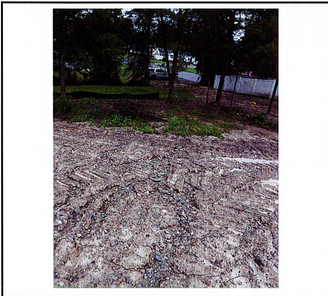
Slopes behind Building 1, 2 and 3 eroded. Open soil remaining idle for longer than 14 days requires temporary stabilization.
