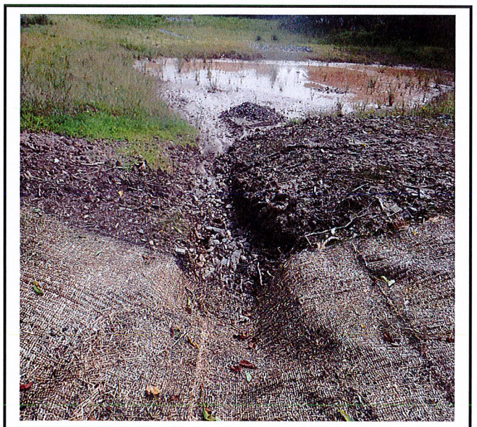
North end drainage swale needs to be re-graded, blanket added and rock outlet protection installed once forebay is cleaned out.
