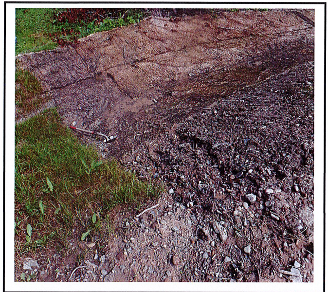
Eroded side slopes of north end drainage channel. All exposed slopes require stabilization.
