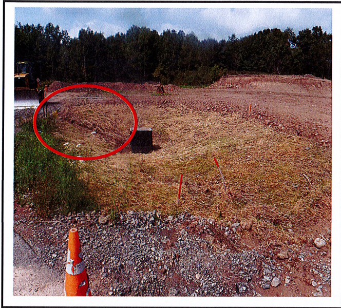
Erosion has started at side slopes leading to catch basin. Re-stabilizing side slopes will prevent further erosion.
