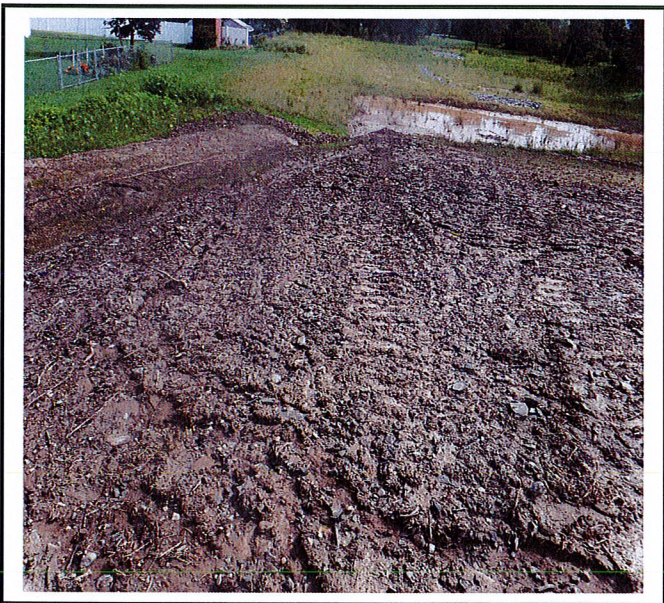
Eroded side slopes of north end drainage channel. All exposed slopes require stabilization.
