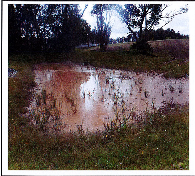
Stormwater forebay completely silted in. It will need to be cleaned out.
