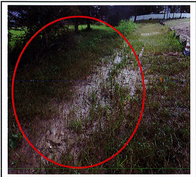
Sediment that went over silt fence has filled the east end drainage swale.
