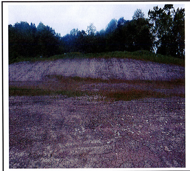
This slope has been stabilized with erosion control blanket but the vegetation is not growing. This slope needs to have grass growing on it because these blankets will biodegrade over time.
