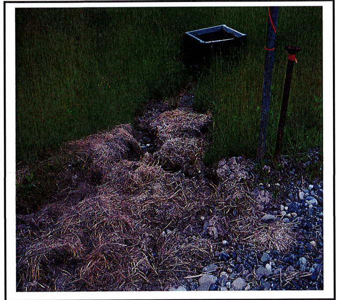
CB 3- Erosion has been occurring here for months. It is not improving but getting worse. Correction is required.
