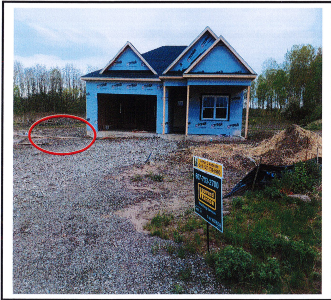
Bare soil requires stabilization.
