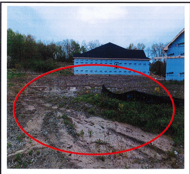
Bare soil requires stabilization. Silt fence should extend further in this area so that sediment does not leave lot.
