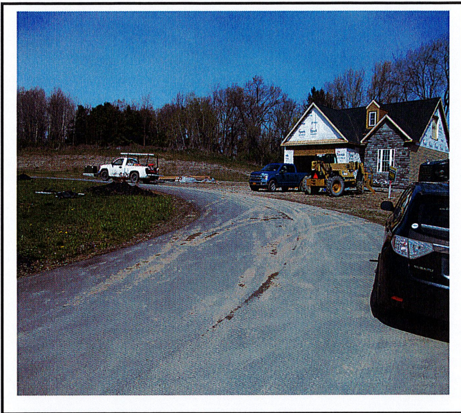
Mud tracked all over the road. Parking along road is disrupting drainage to infrastructure.
