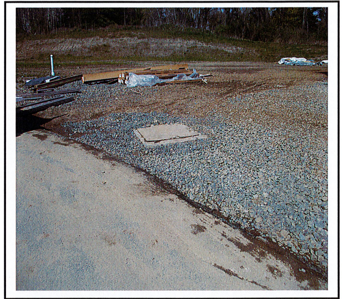
Driveway constructed around existing catch basin. Catch basin has no sediment control practice to prevent sediment from getting into system.
