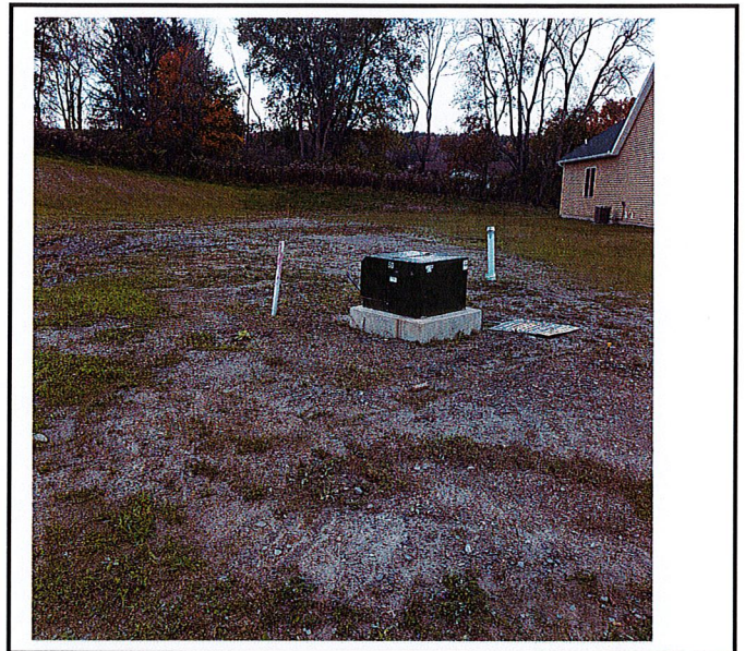
Compacted areas will not grow grass. Decompaction and stabilization required.
