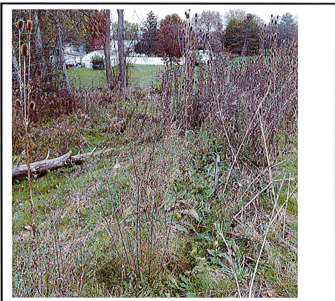
Silt fence is installed in those weeds across the drainage swale. It must be removed.
