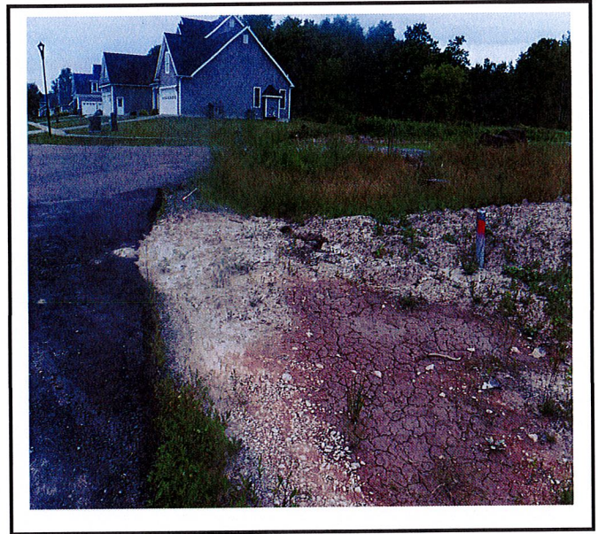
Exposed soil needs to be stabilized.
