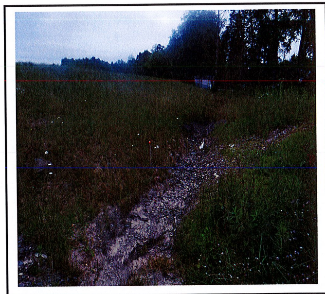
Headcutting is still occurring at the discharge outlet of the drainage swale. Sediment is depositing into the pond.
