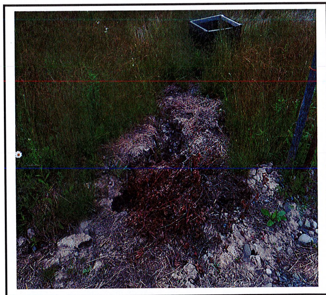
Erosion is still occurring around CB-3. Also, yard waste is in the eroded area now.
