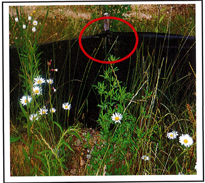
Silt fence has reached its lifespan and requires replacement.
