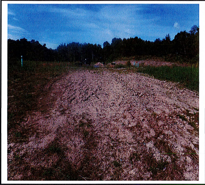
Graded area on Lot #4 leading down to stormwater basin is showing signs of erosion. Stabilization is required.
