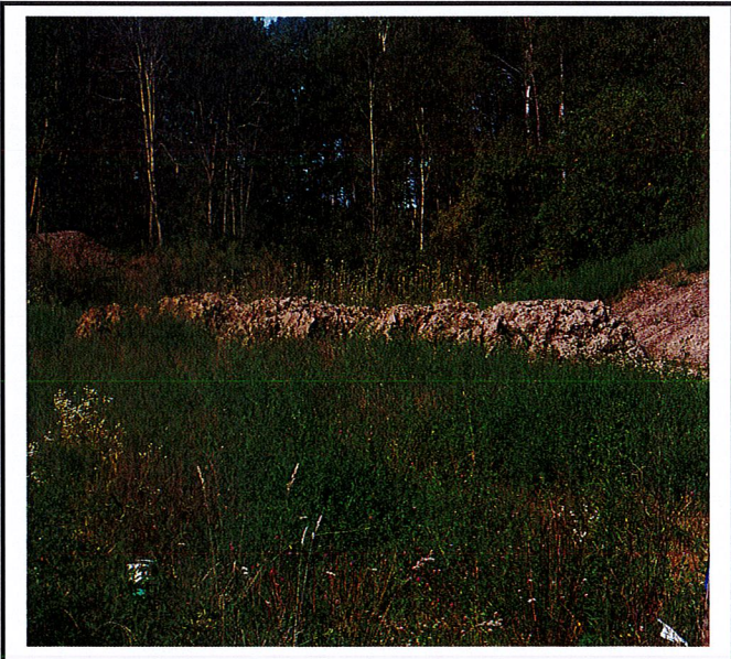
Stockpile of material removed from stormwater basin requires stabilization.
