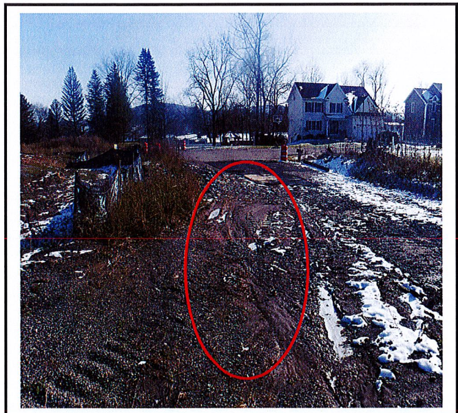
Sediment being carried off Lot 9
