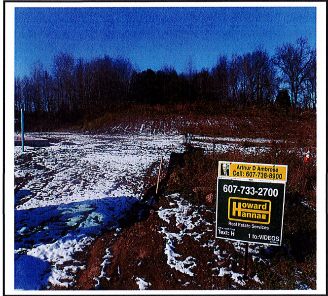
Lot 9 needs construction entrance and erosion and sediment control around entire lot.
