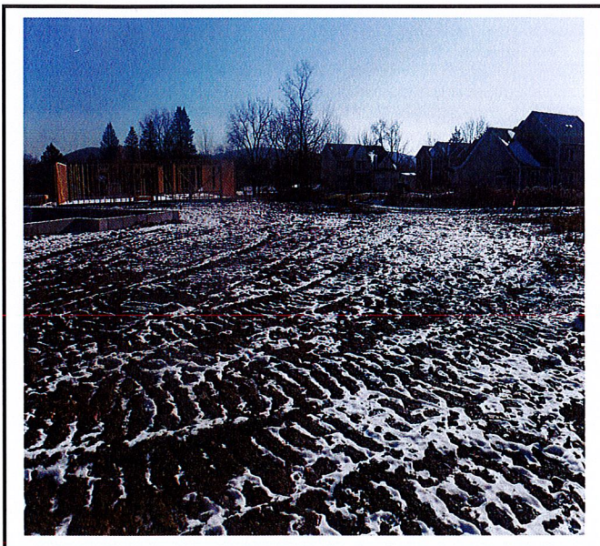
Back end of Lot 9 has no erosion and sediment controls.
