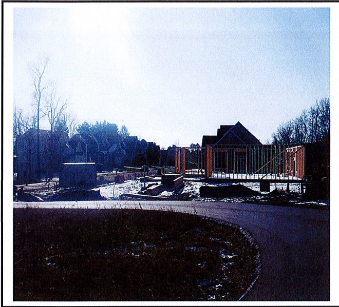
Silt fence needs replacement and repair all around Lot 10.
