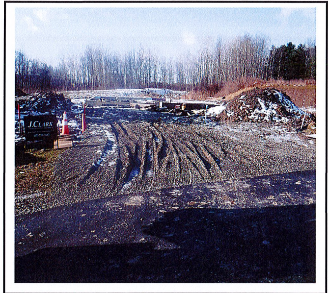
Topsoil pile needs to be stabilized. Construction entrance needs maintenance.
