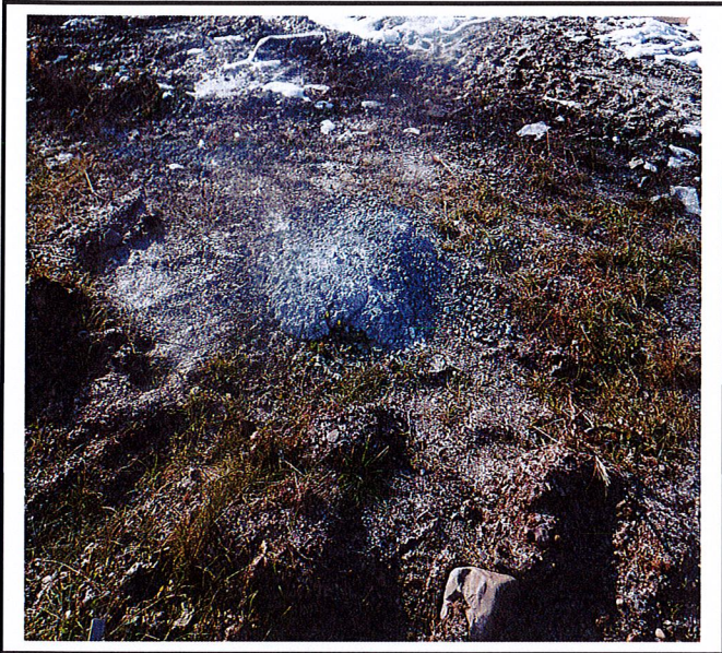
Concrete washed onto the ground. Concrete washout needs to be installed.
