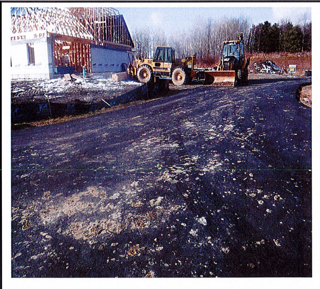
Construction entrances on both open lots need maintenance.
