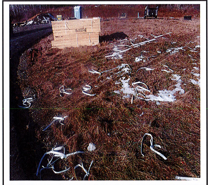
Garbage and debris around site needs to be cleaned up.
