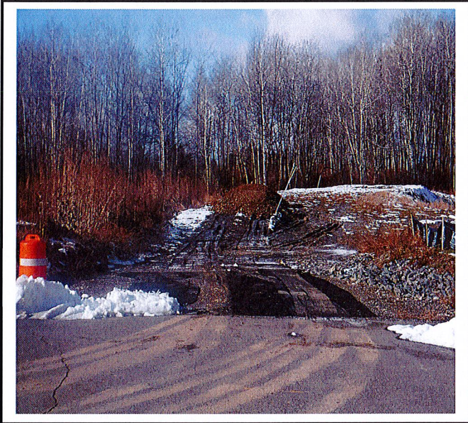
Mud is being tracked onto Lynhurst Ave from fill being dumped on future road. Construction entrance needed.
