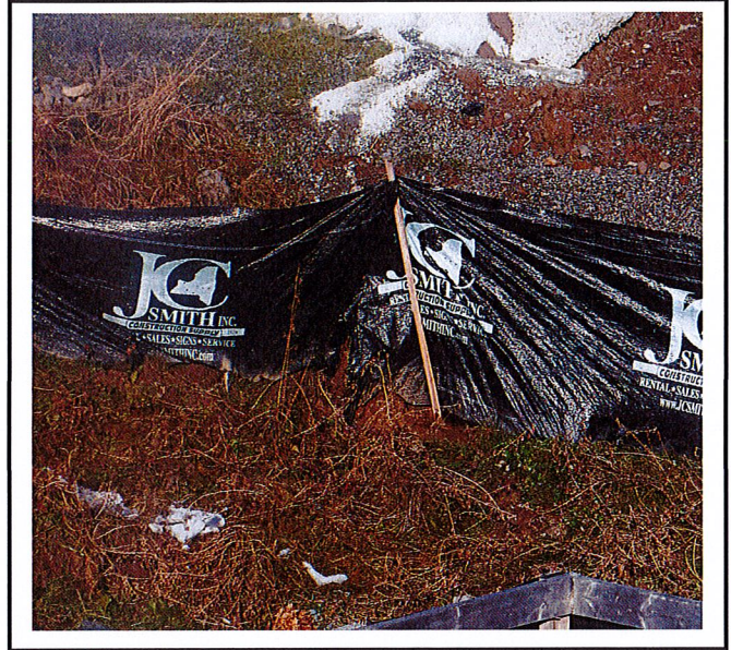
Silt fence requires maintenance and repair around the entire site.
