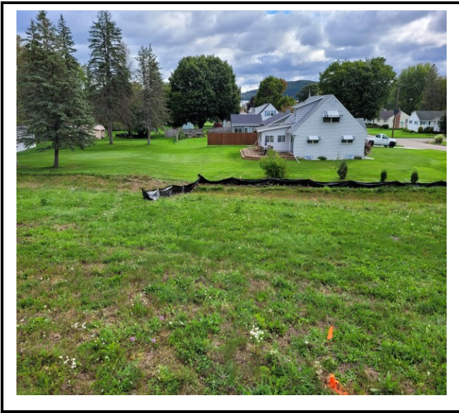
Silt fence is located across the drainage swale which is not approved at time of visit.
