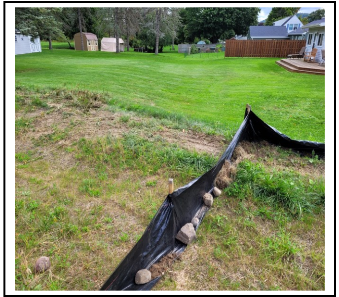
Silt fence crosses drainage swale. Silt fence does not belong in concentrated flow areas.
