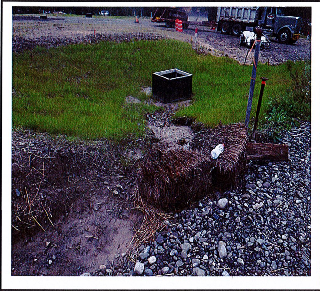
Erosion occurring down to CB3. Straw bales are not an accepted practice for erosion control and as you can see caused more damage and erosion.
