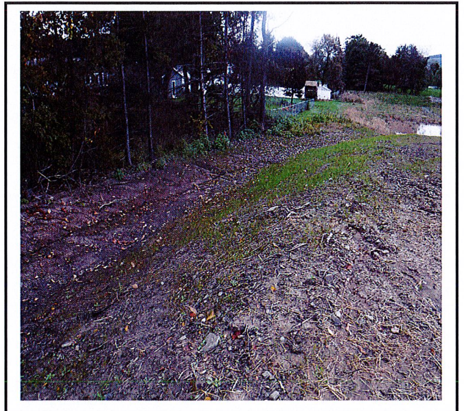
Drainage swale has not been corrected yet.
