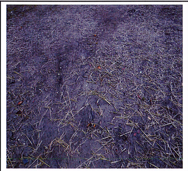
Mulch rate does not meet NYS standards (2 tons per acre) and because this project will be open in the winter the site must meet winter rate of 4 tons per/ac.
