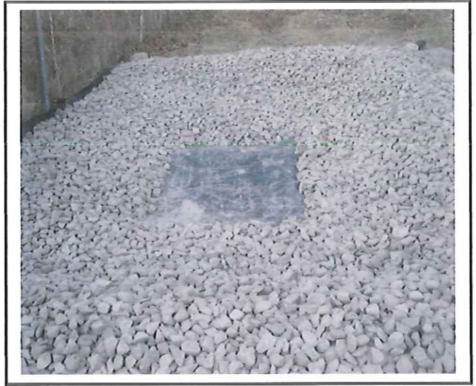
Drop inlet protection-stone placement is good but the wrong fabric material was used. Water will not flow through this.
