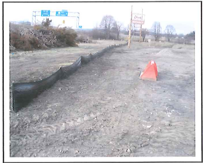
Silt fence and disturbed area along I-86 West.
