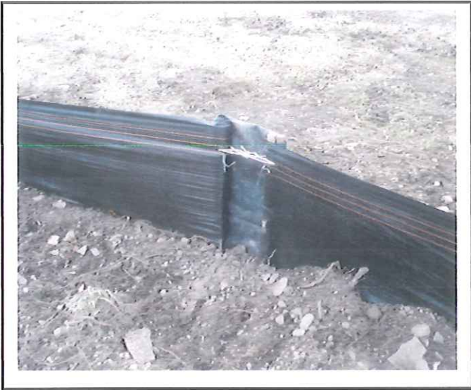
Correction made to each gap in the silt fence.
