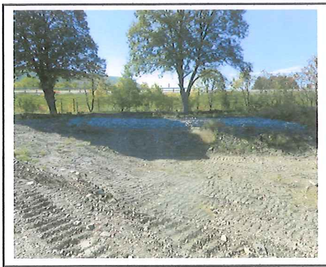
All open exposed soil needs to be temporarily stabilized.
