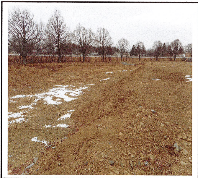
Stormwater basin appears to be over excavated.
