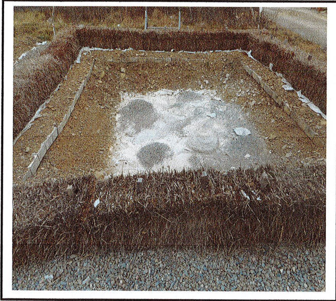
Concrete washout requires maintenance before the next scheduled concrete pour.
