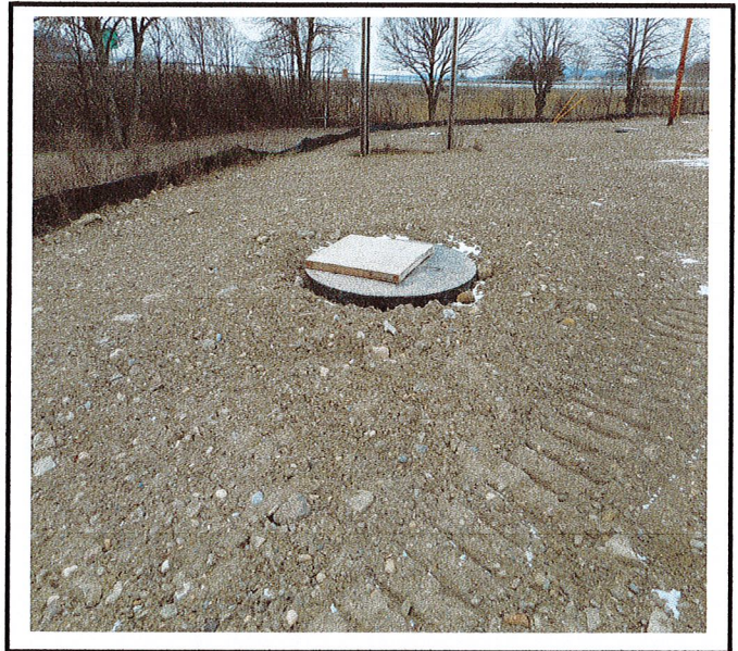
Soil exposed and not stabilized. Drop inlet protection not installed at any of the catch basins.
