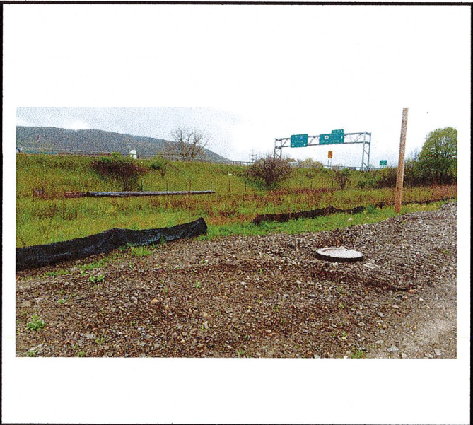
All silt fence needs to be replaced.
