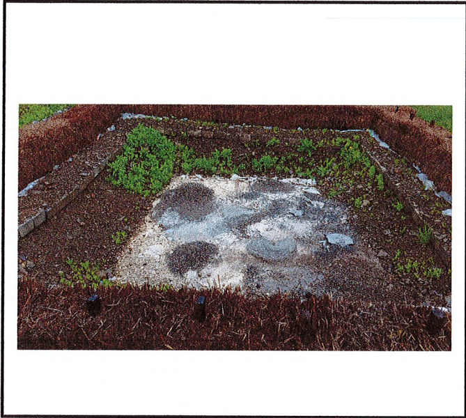
Concrete washout needs to be maintained.
