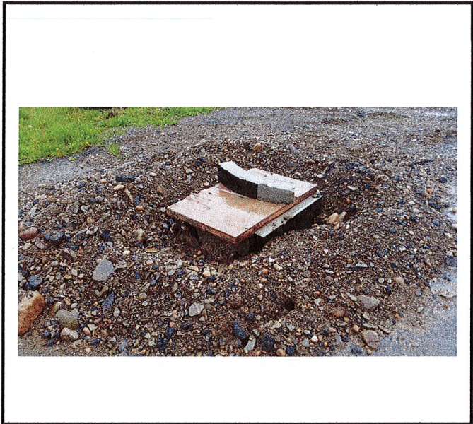
All catch basins require the correct erosion and sediment control protection.
