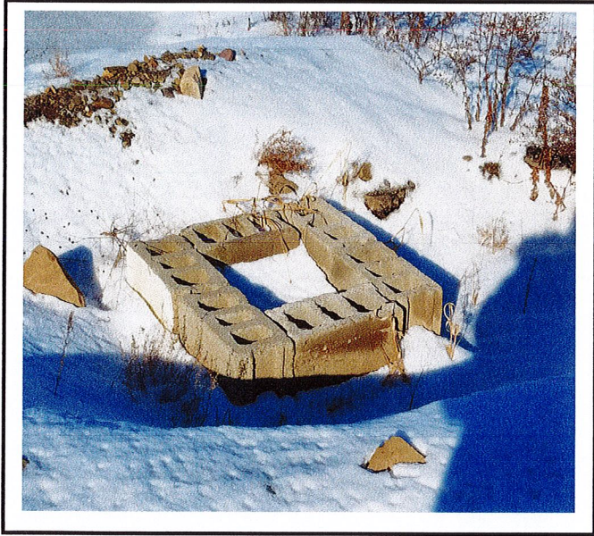
Drop inlet protection not installed correctly.
