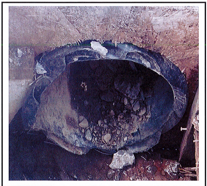
Storm sewer inside catch basin- evidence of soil and sediment laden water in pipe.
