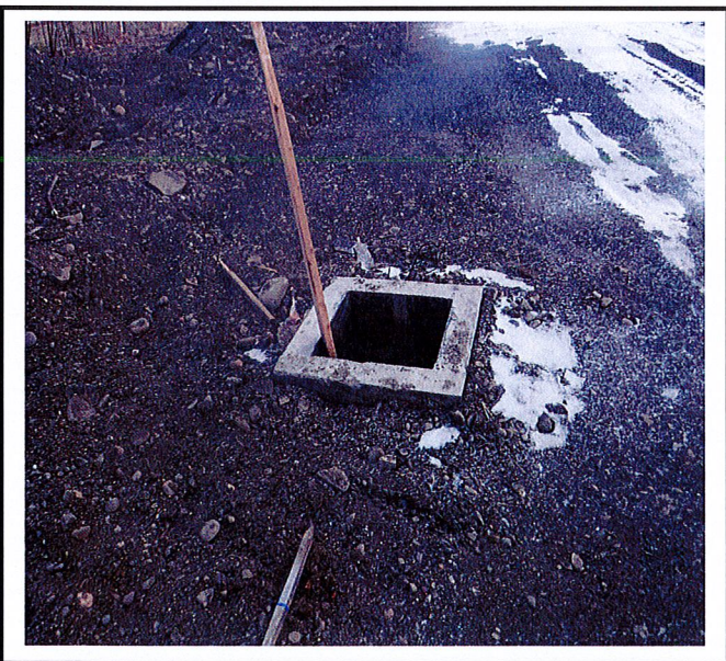
Catch basins along north end of property are at grade and receiving soil and debris. Protections are required.
