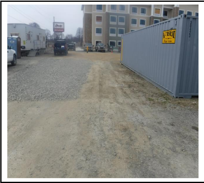
Construction entrance is correct but traffic can go around it. Monitor to ensure that traffic doesn't track mud.
