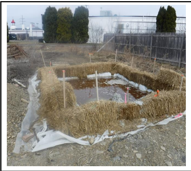
Concrete washout is at capacity and needs to be replaced before the next pour.
