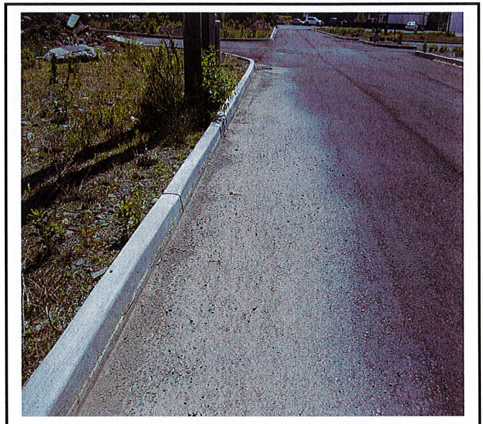
Sediment laden water is getting into the storm sewer.
