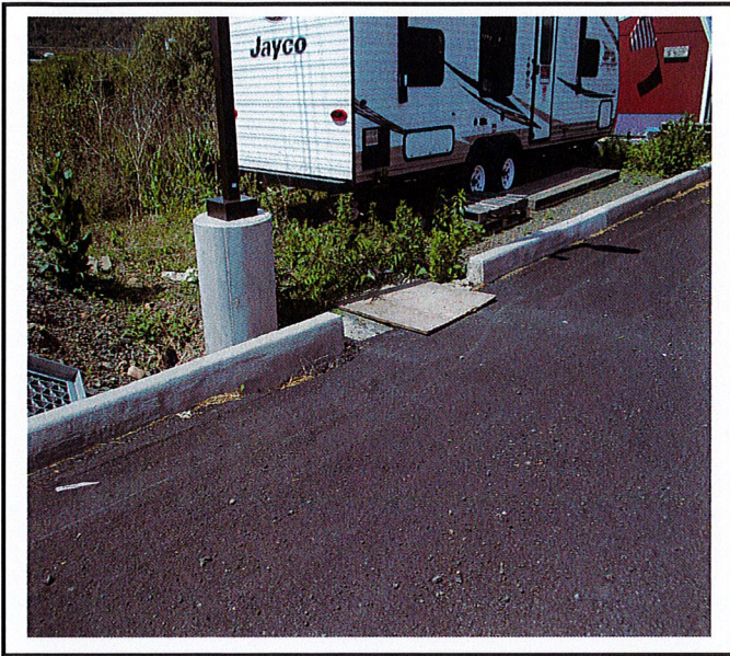
Concrete curb is not directing stormwater to the catch basin (under plywood).
