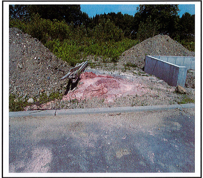
Concrete washed onto the ground.
