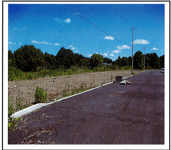
Open soil needs to be stabilized and stormwater basin protected from sediment.
