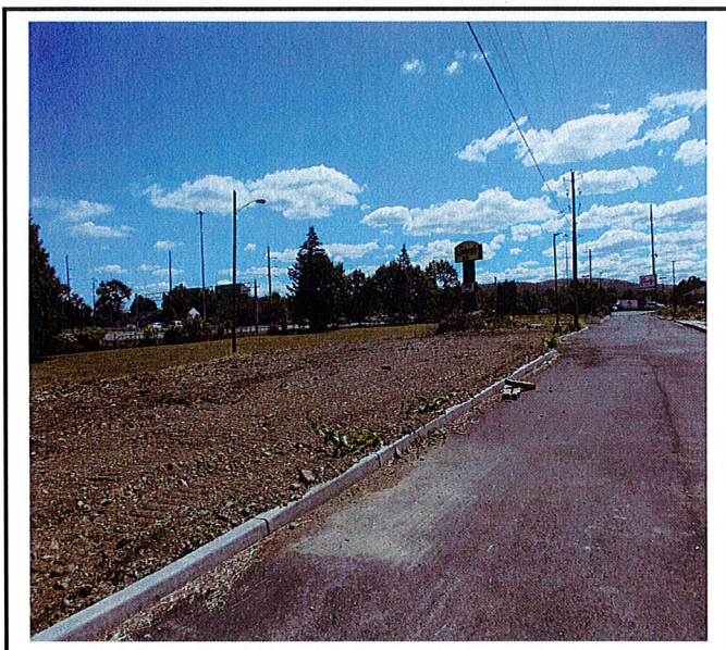
Open soil needs to be stabilized.
