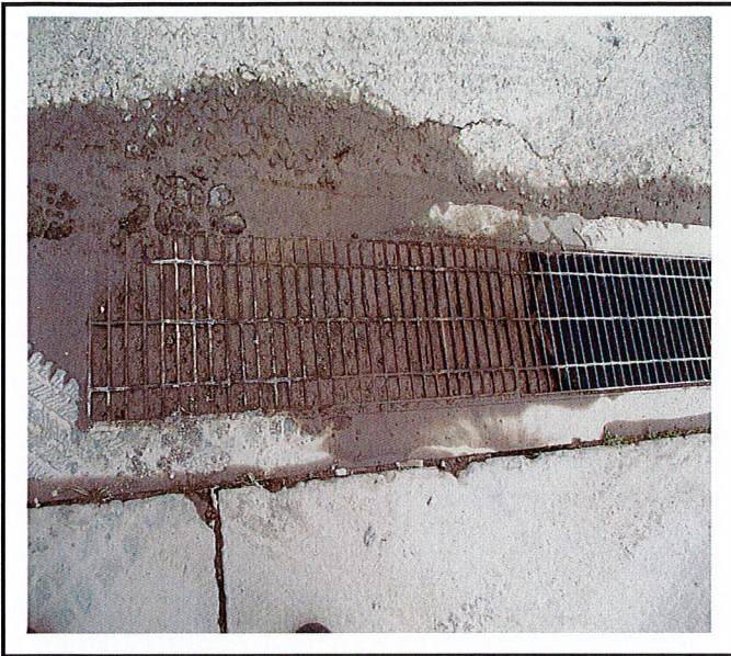
Trench drain in parking area is filled with sediment from project erosion/runoff.
