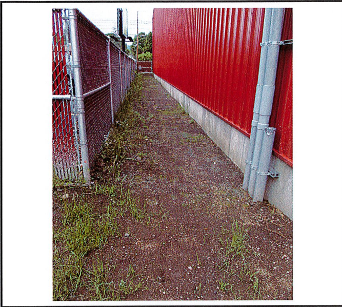
Area along south end of building requires soil stabilization. Soil needs to be covered with mulch.
