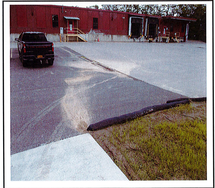
Sediment barrier needs to be wrapped up towards concrete to hold back sediment. Sediment filled trench drain in parking lot.
