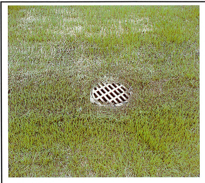
Sediment bag insert will need to be removed from the south dry well in swale along College Ave. once 80% vegetation is established.
