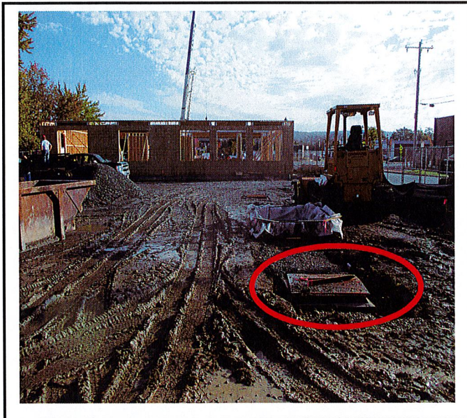
Catch basin drainage structures require protection spelled out in approved SWPPP.
