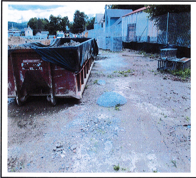
Concrete washed onto ground.
