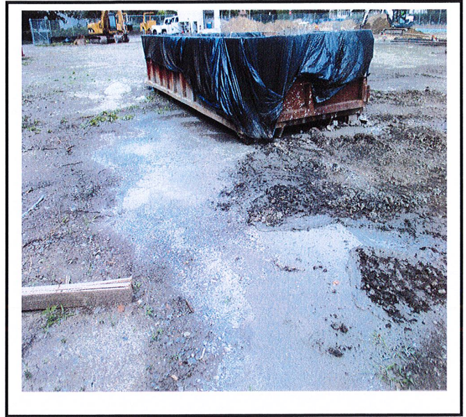
Concrete washout is not functioning properly.
