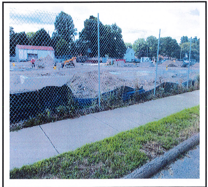
Silt fence around the project area needs to be repaired as foundation is backfilled.
