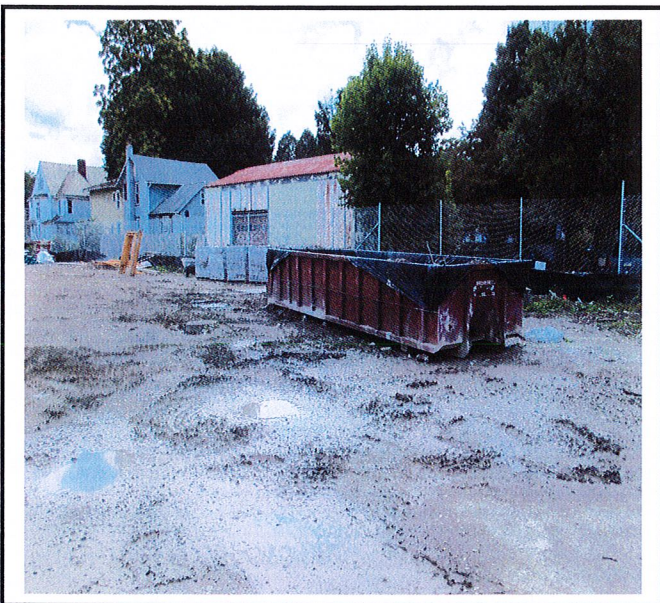
Concrete washout is not functioning properly.
