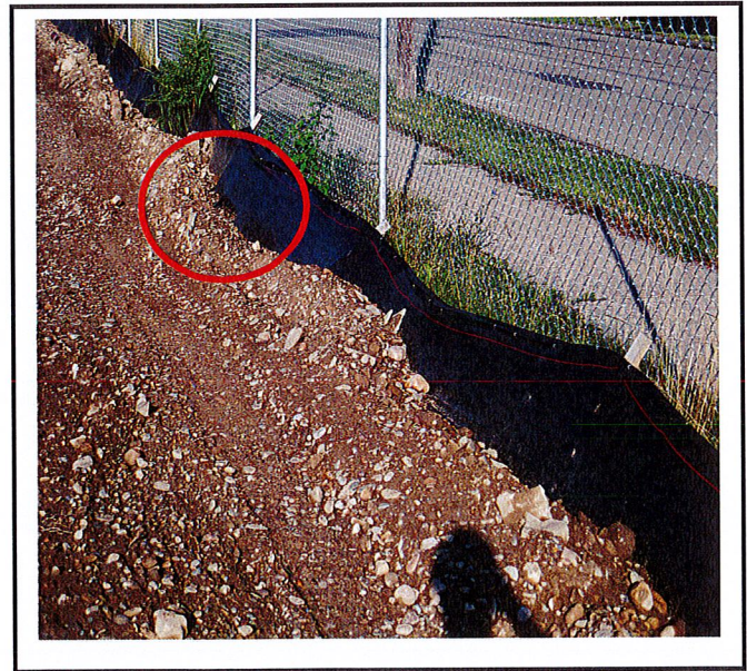
Silt fence has holes in it. It is being encroached upon with traffic around the building.
