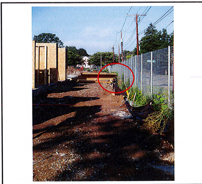
Silt fence is requires maintenance. It is down in some areas, encroached on in others and the building panels are on top of it in other locations.
