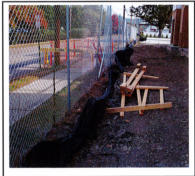
Silt fence around entire site is in disrepair.
