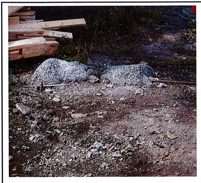
Concrete washed onto the ground.
