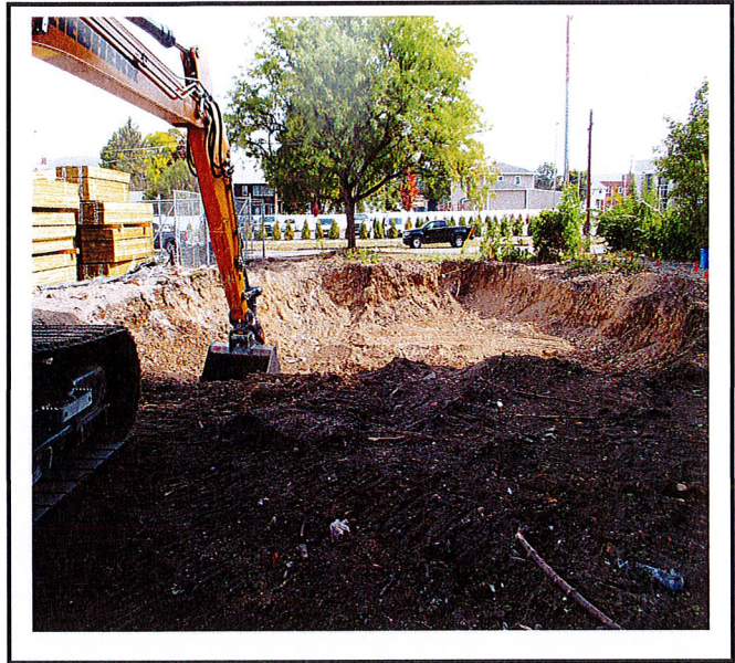
Work has started in new area of project and no erosion and sediment controls are installed.
