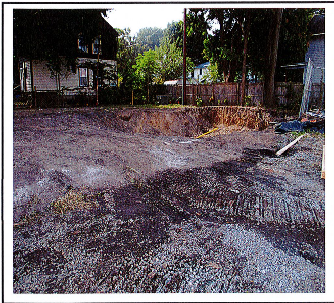
Work has started in new area of project and no erosion and sediment controls are installed.
