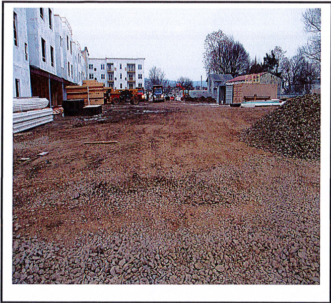
Construction entrance needs to be replaced. Stone is on site to install.
