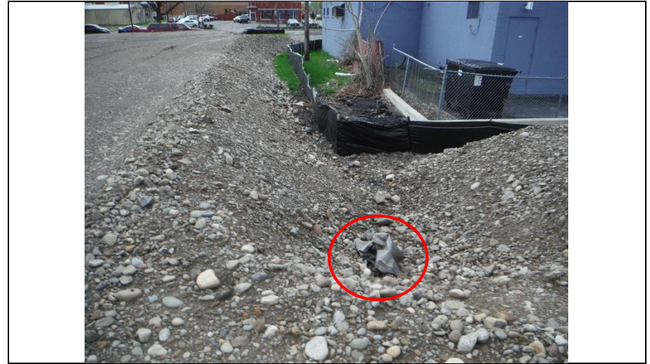
2.) Unacceptable stormwater inlet on western side of property facing south (corner of existing Savino's Liquor).
