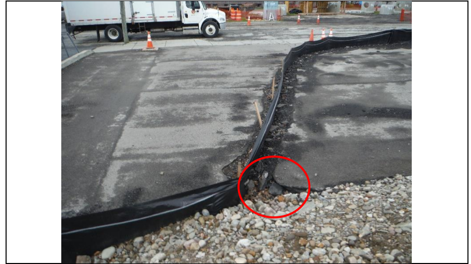
6.) Silt fence off wood stakes. Western side of property facing west. Just north of Savino's Liquor.
