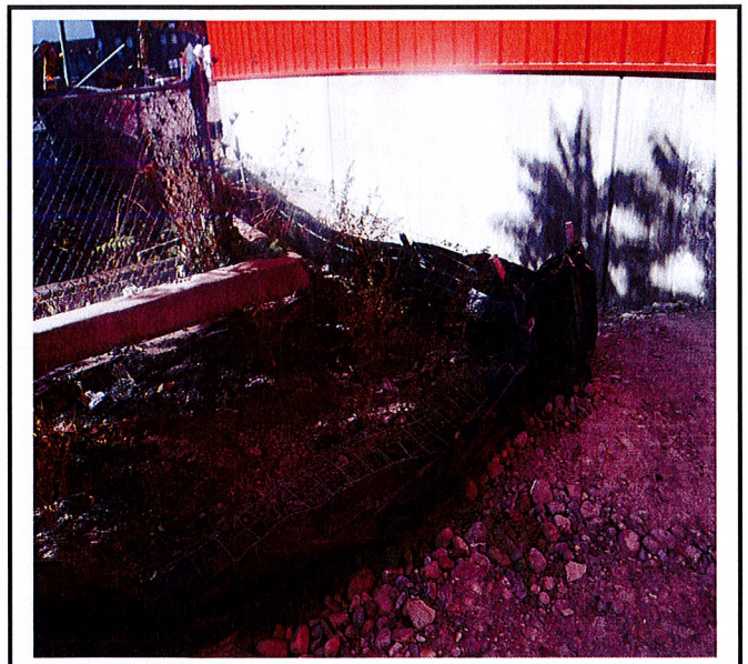
Silt fence needs to be maintained around the entire project site.
