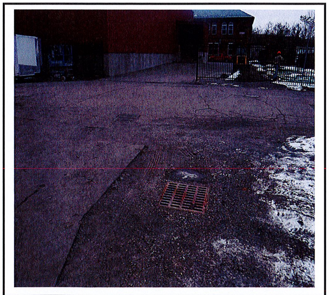
Unprotected catch basins from S. Magee Street and W. 3 rd Street.
