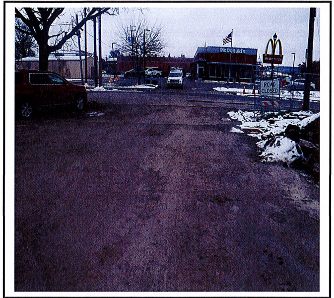
No construction entrance is installed and sediment is getting tracked off site onto W. 3 rd street.
