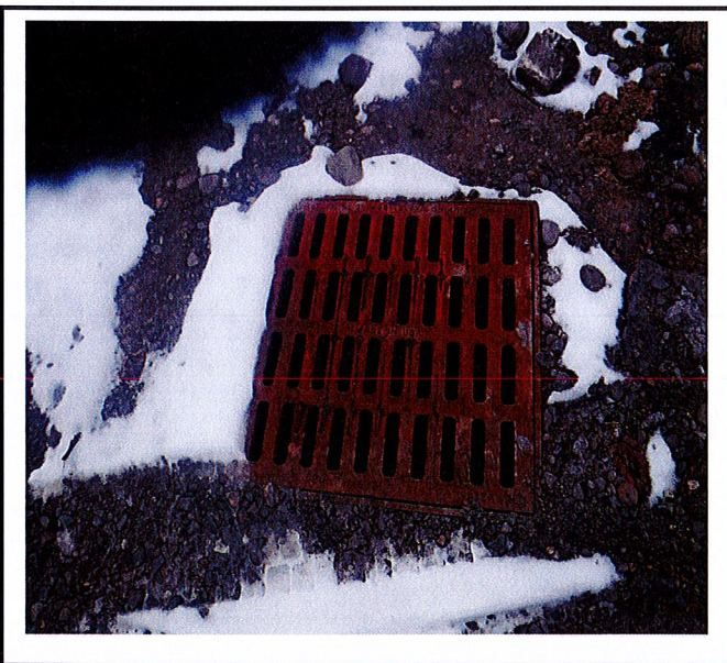
Unprotected catch basin near construction trailer and W. 3 rd street.
