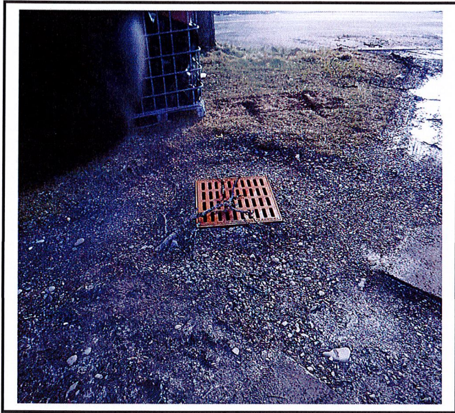
All catch basins need to have inlet protection installed. There are 3 catch basins total.
